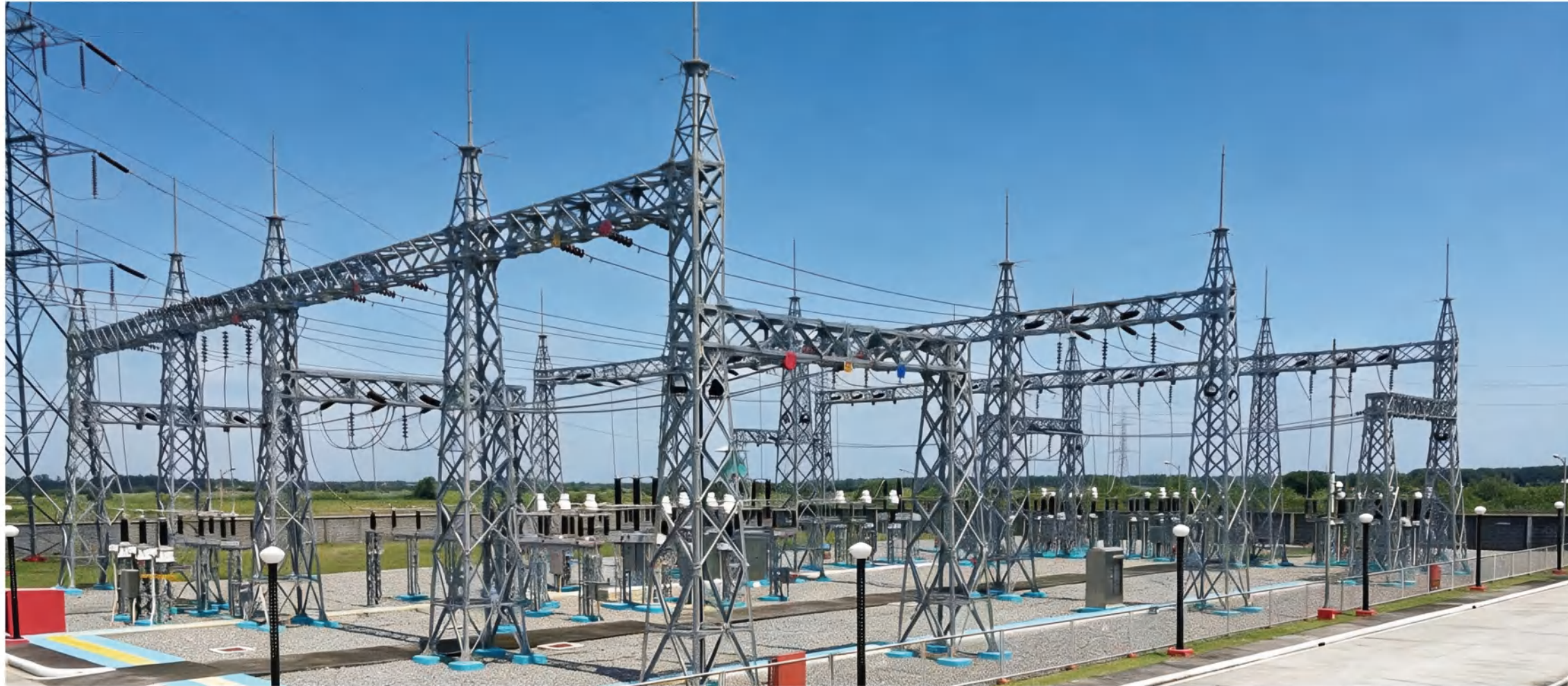
© 230 kV San Esteban Substation Expansion in the Philippines
