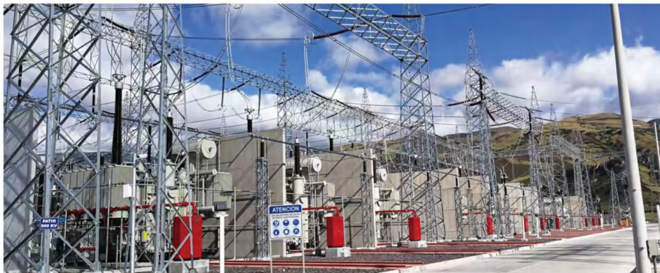
500kV, 200MVA single-phase high-capacity transformer at the Inca Substation in Ecuador
