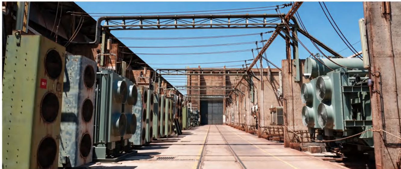
© Specialty transformer project for the Metlen aluminium plant in Greece
