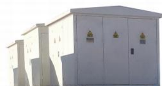
Compact (pad-mounted) substation (Including wind power and photovoltaic)
