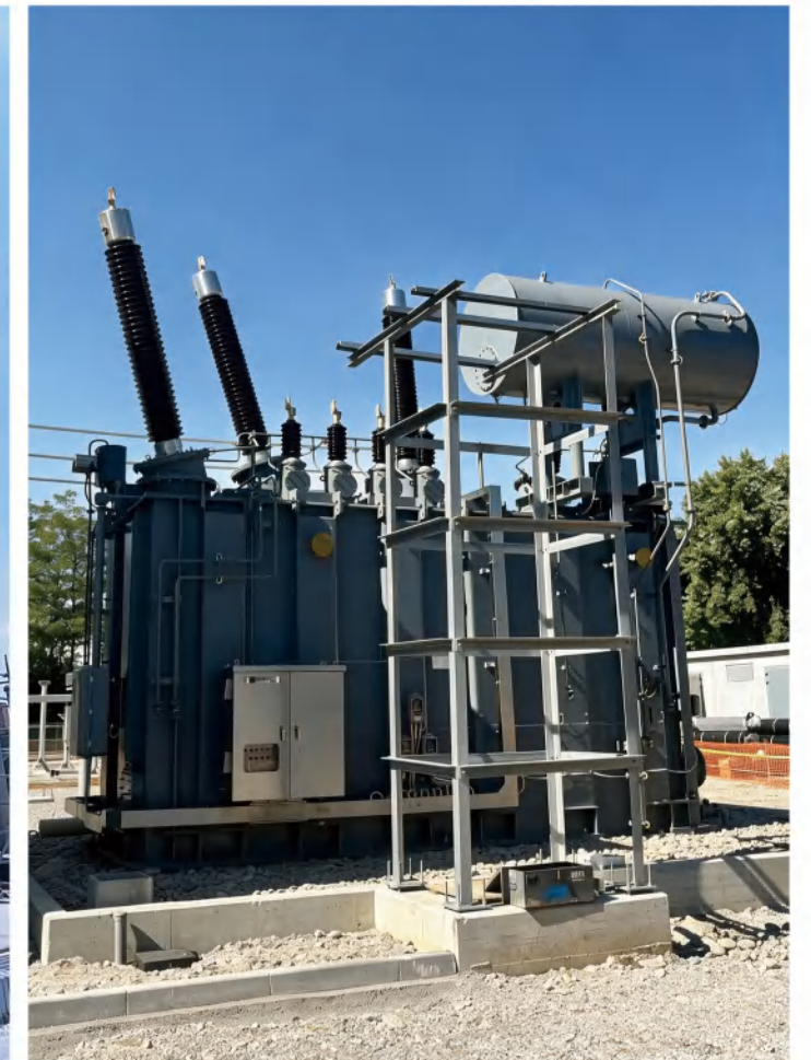
Transformers for the Substation at the Conexus Milan Data Centre in Italy
