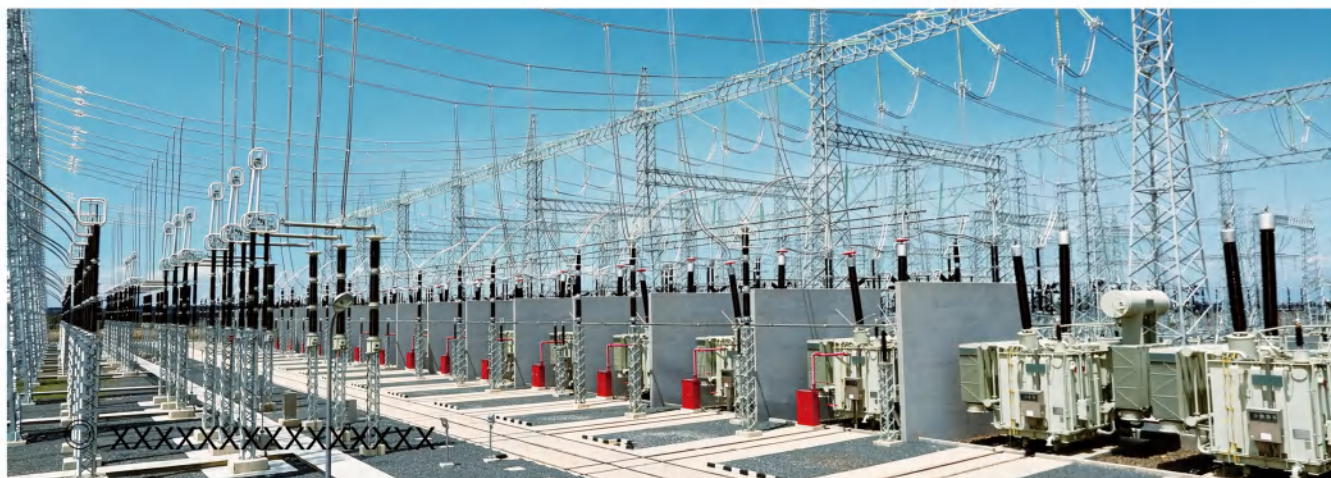
© Delivered 23 × 500 kV and 8 × 400 kV power transformers.
